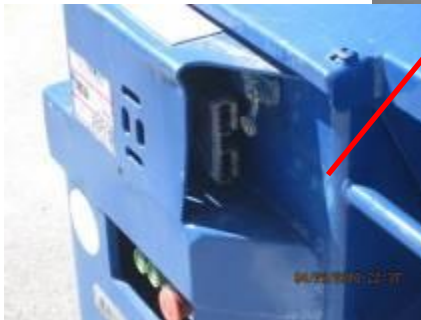
Battery Charger Connection
